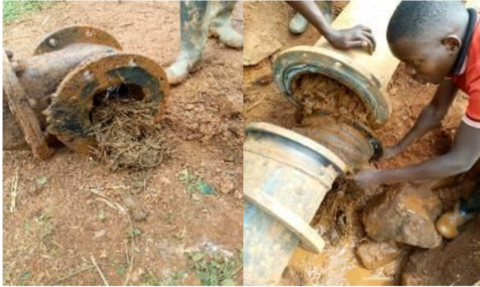
Photo 127. Sediments in valves at the middle of pipeline and The pipe was full of sediment at the starting point
