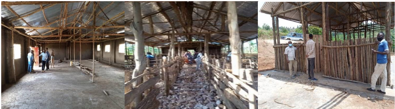
Photo 78: Pig and chickens houses construction by the group participation for both women and youth
