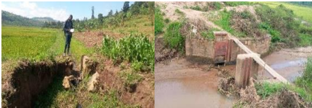
Photo 112: Nyabuyogera irrigation infrastructure status
