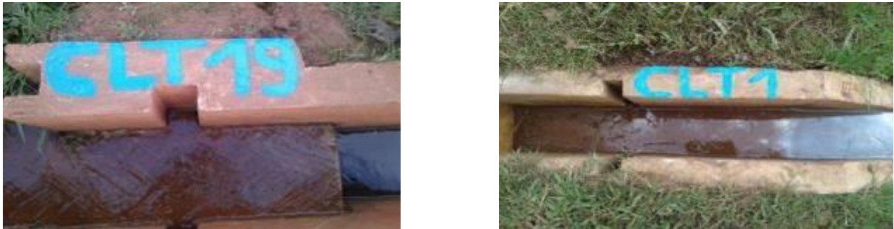
Photo 144. Examples of coding facilities in Cyimpima scheme
