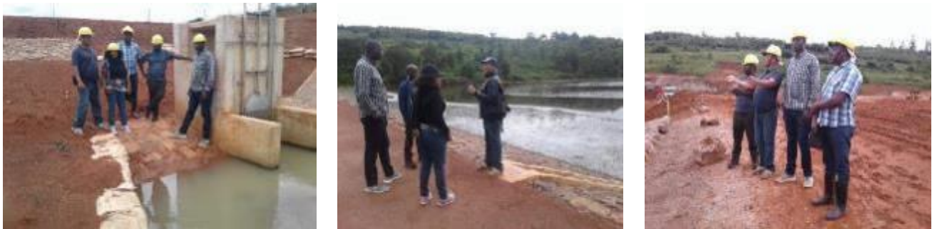
Photo 140. Field visit with Core C/Ps/RAB in Cyimpima, Gashara and Bugugu schemes under construction
