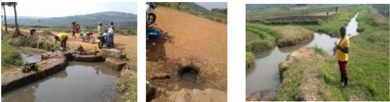
Photo 145. Culvert in Cyaruhogo, Culvert crossing road and Junction of Gashara and Cyaruhogo drains
