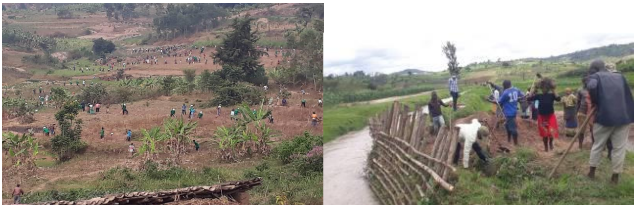
Photo 102: Community work in Ruhango, near Base (left) and repair of damage at Base scheme (right)
